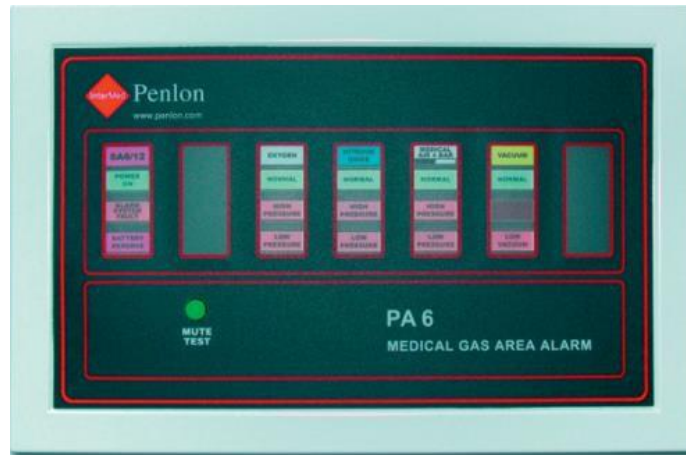
FIGURE 7-9 Medical gas alarm panel.
