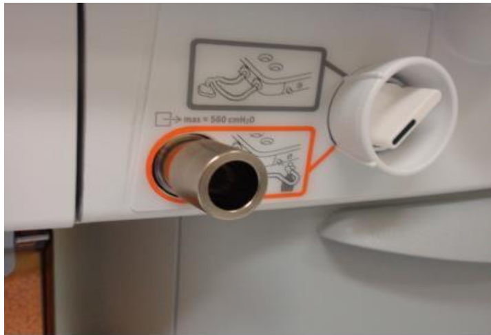
Fig. 8.29 Common gas outlet
