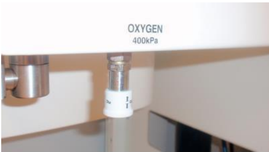
Fig. 8.26 Compressed oxygen outlet
