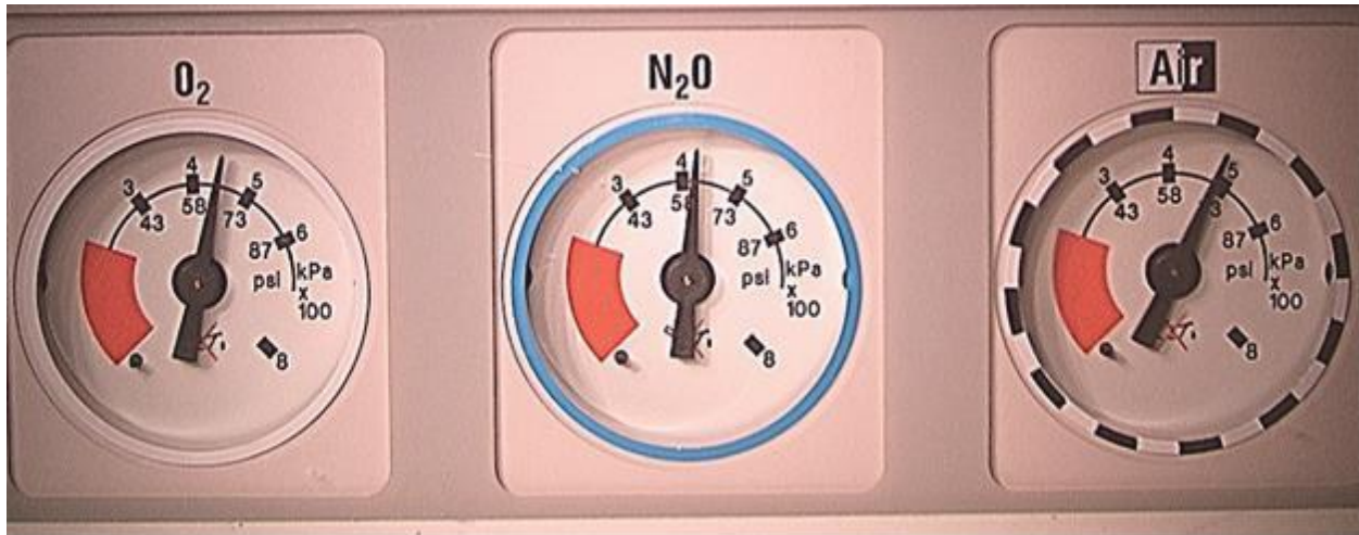
Fig. 8.3 Pipeline pressure gauges for oxygen, nitrous oxide and air.
